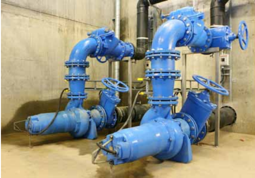
Pumps for waste water Århus creek (Rotan)
